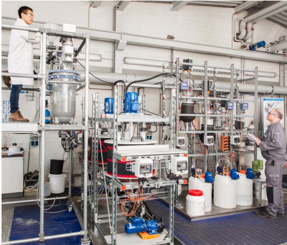
Fig. 3 Treatment of eudialyte concentrate was performed in the demonstration pilot plant at the IME Process Metallurgy and Metal Recycling lab of RWTH Aachen.
