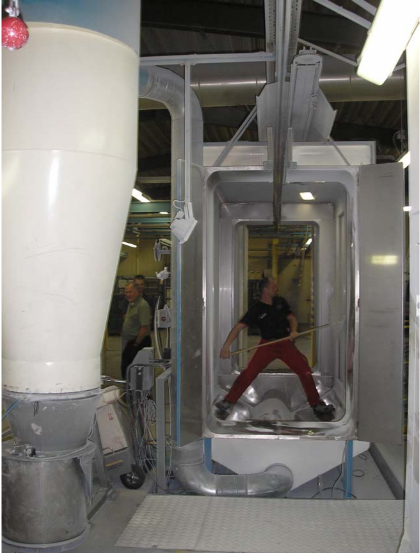
Fig. 1: Automatic spray cabin at NWO
