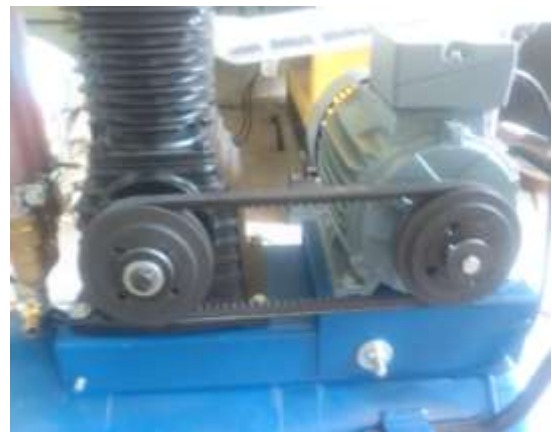
Figure 11: Compressor with changed wheel
