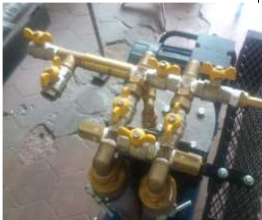
Figure 10: Overview of the installation
