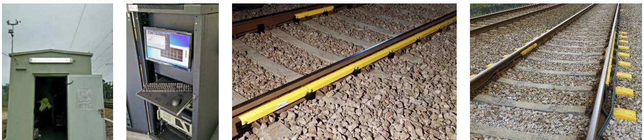
Figure 3 - Wayside system in Portugal: data processor unit and system installation in the track
