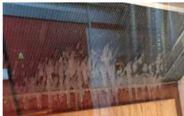
Figure 15: Icicles at the outlet of the heat exchanger with anti-ice coating.
