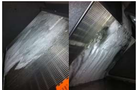
Ice formation on air fins from EXHAUSTO A/S heat exchanger.
