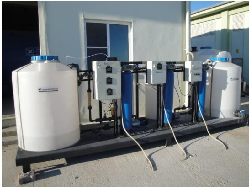
Fig.16 Pilot plant with three filter units (Denizsu, Konya)
