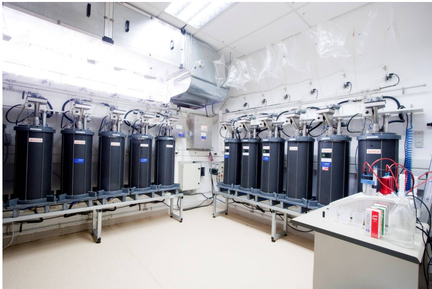
Figure 2.1. AINIA's pilot digesters used for the study of the VFAP evolution depending on the feed.
