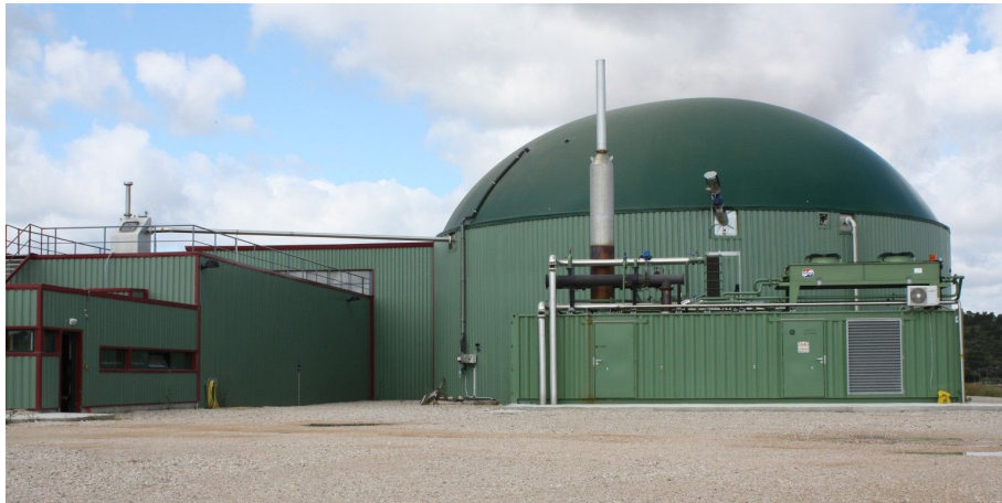
Figure 5.1. Biogas plant of the partner GSR where the prototype was installed and validated
