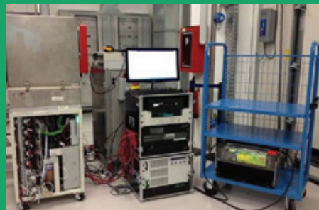
Initial tests on the SOFC module and battery electrical integration.
