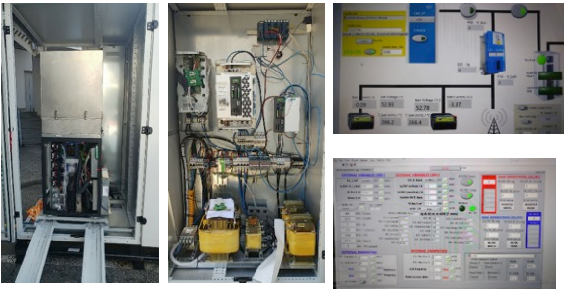
Figure 26: The developed sheltered system: SOFC generator, power conversion compartments and software interface
