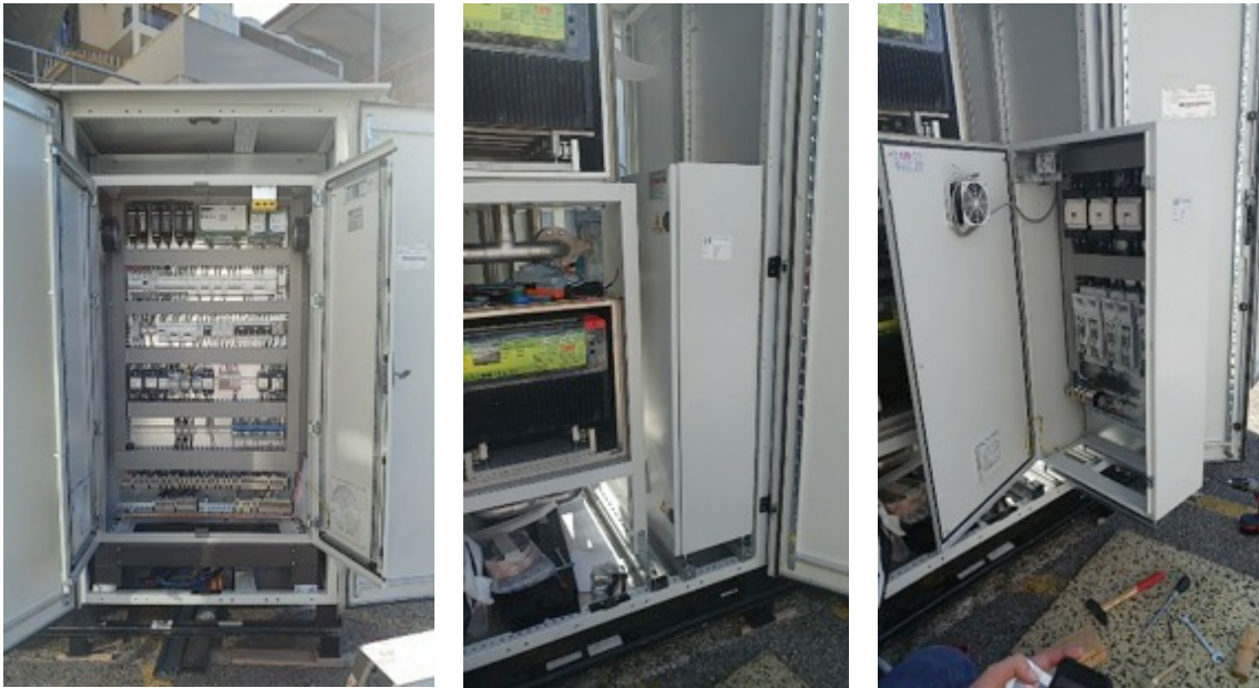
Figure 25: The developed sheltered system: control equipment and SNC batteries compartments
