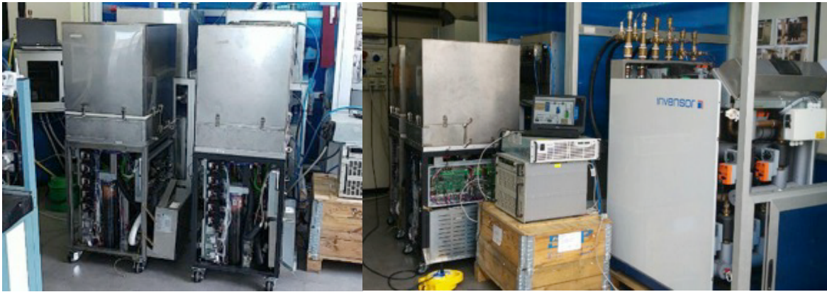
SOFC sub-systems installed and connected with the SNC batteries
