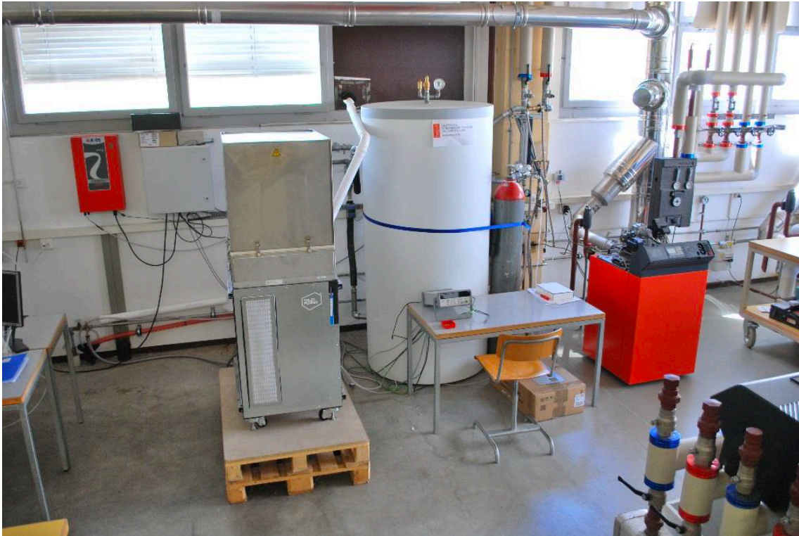
Figure 18: The first SOFC generator delivered and installed at HEIG laboratory in Yverdon (CH)
