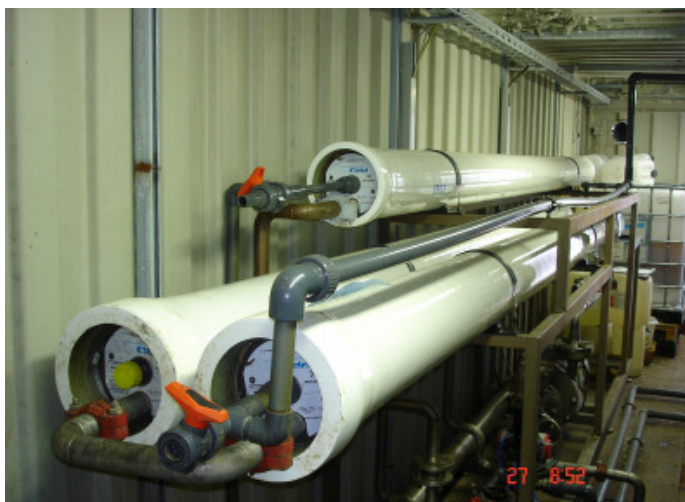
Figure 5: Reverse osmosis unit of 2 step membrane filtration plant
