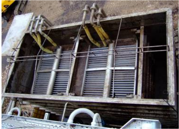
Figure 6: External filtration unit of the membrane bioreactor plant
