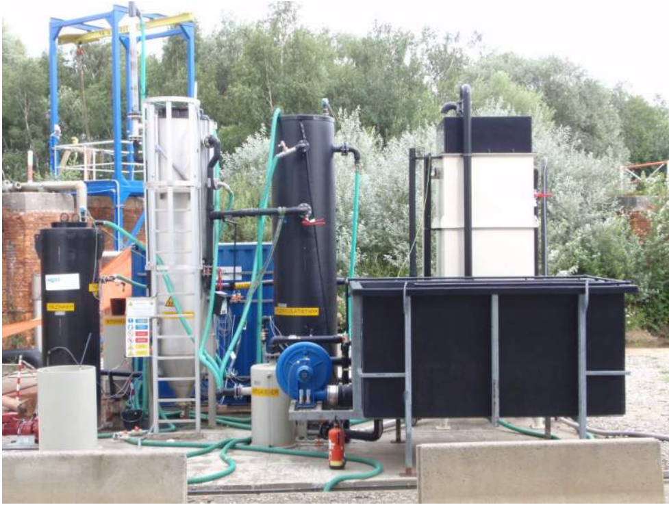
Figure 23: Installed pilot plant at the Umicore Hoboken site in Belgium.
