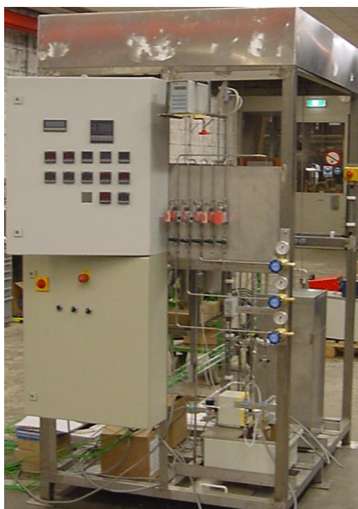
Figure 9: High temperature gas cleaning system
