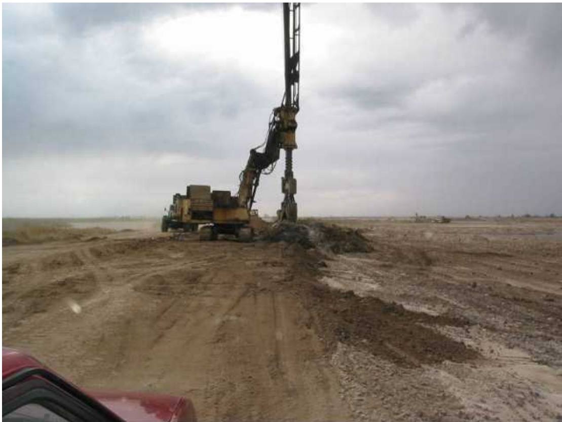
Fig.19. Construction of anti-filtration screen, so called cut-off wall around mercury waste lagoons
