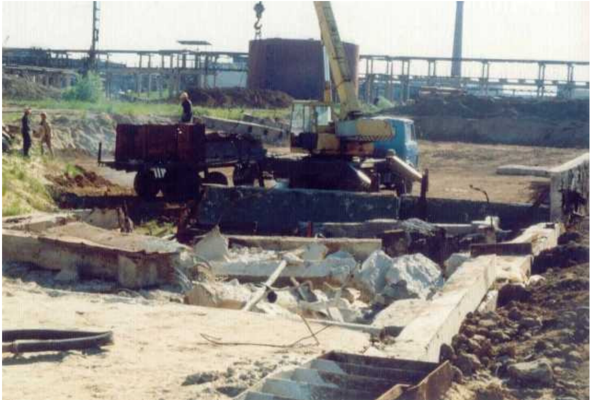
Fig.22. Piling mercury contaminated building structures into the third compartment of the landfill
