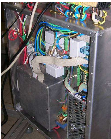
Figure 18: Internal view of the electronics - MCU board shielding and general layout.
