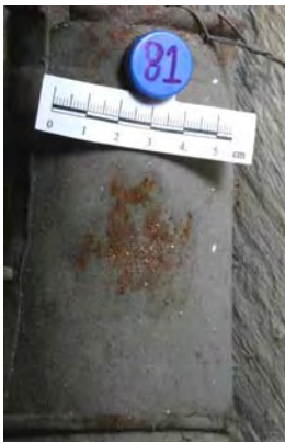
Figure 1 Localised corrosion on an artifact exposed on the wall.
