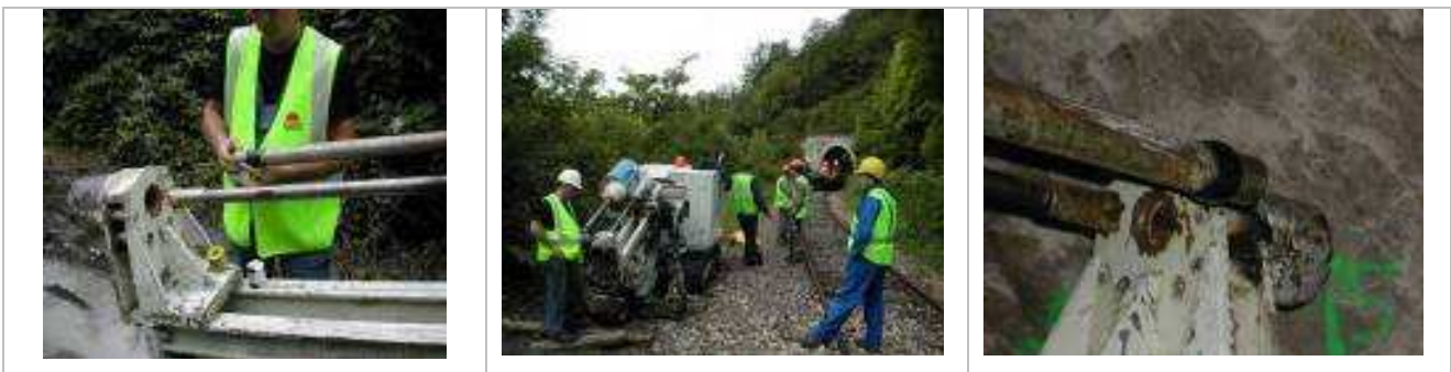
Figure 14 - Field Tests on NiTi reinforced collar on Ditta Ripamonti equipment in Frejus
