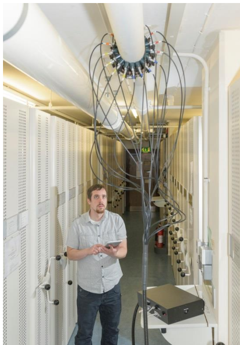
Figure 6. SprinkTest integrated system.
