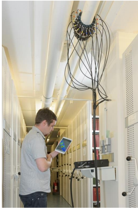
Figure 5. SprinkTest integrated system.
