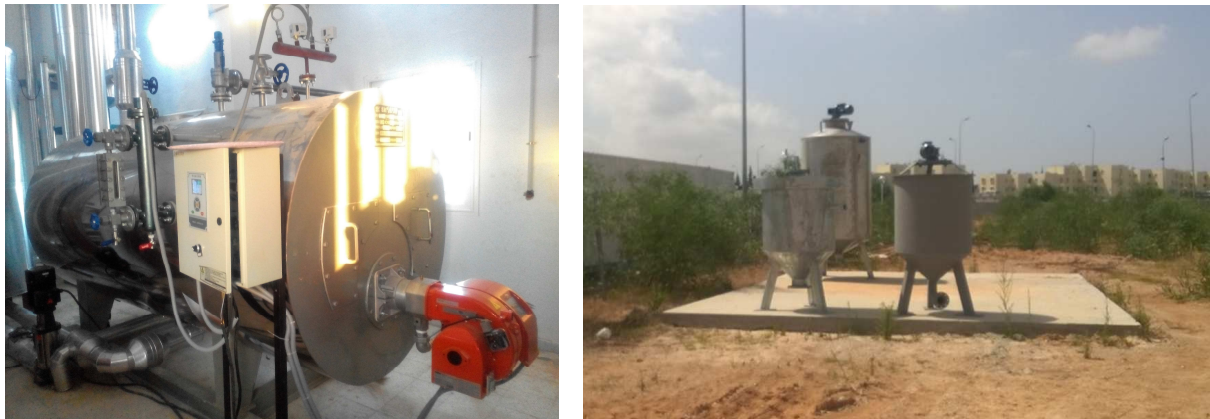
Figure 17. View of biomass boiler (left) and biomass digestion sub-system units (right).
