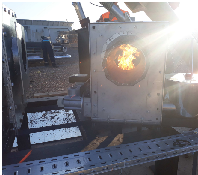
Figure 13. View of biomass combustion in the boiler.
