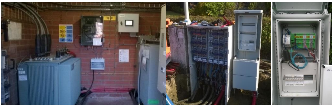
Figure 13: Substation with OLTC (left) and cable cabinets with measurements and communications (right)
