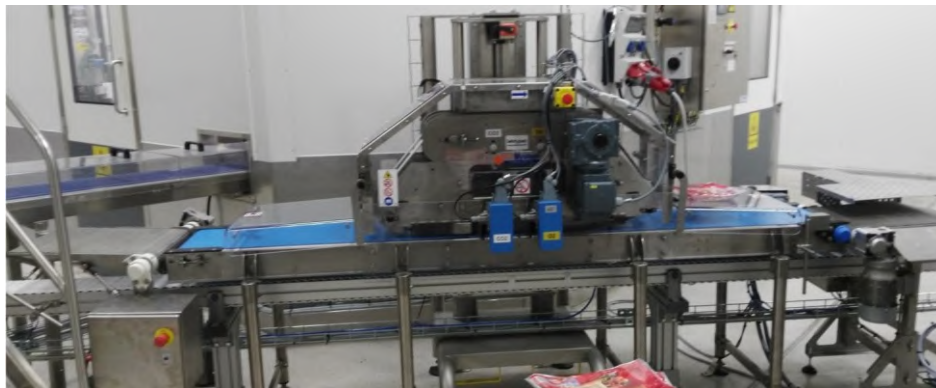
SAFETYPACK machine: In-line version installed at Santa Maria plant.
