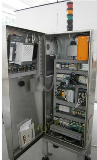
Control Panel: electrical cabinet and industrial PC.
