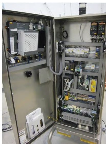
Control Panel: Electrical cabinet and industrial PC
