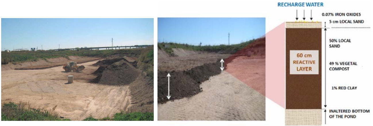
Fig. 8: Construction of the infiltration pond at the Llobregat river in Barcelona (left), and set-up and composition of the reactive layer (right).
