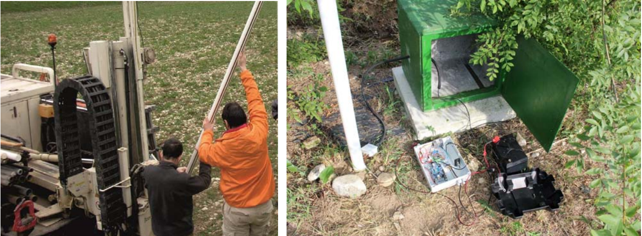
Fig. 11: Installation of waveguides for the TDR system using direct push equipment (left), and connection of the waveguides to the TDR system that were housed in a box on-site for permanent data recording (right).
