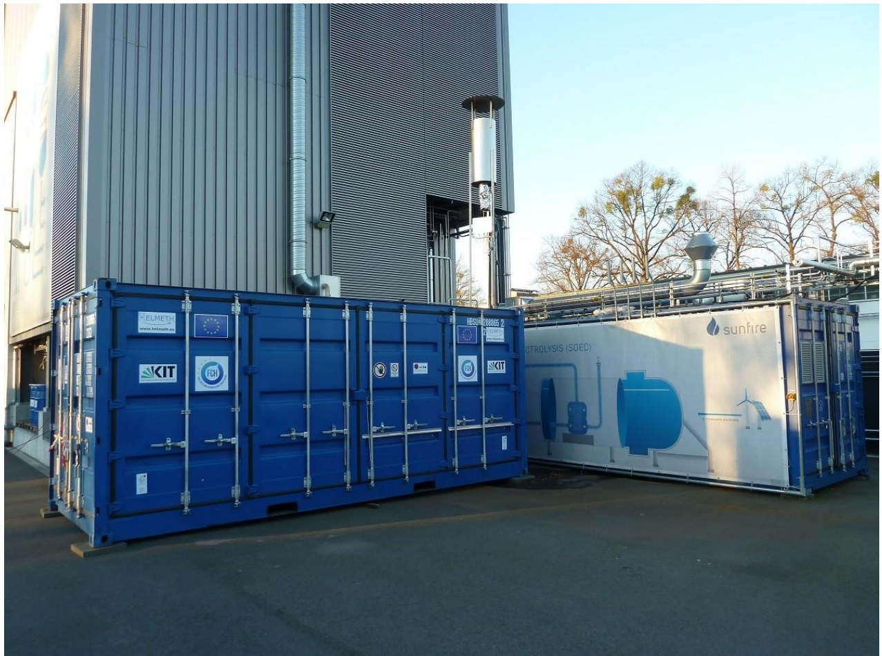
Figure 8: Coupled PtG plant (left container: methanation; right container: electrolyser)
